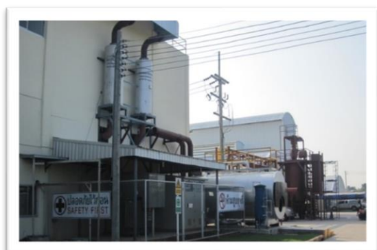
Biomass Power Plant- Satake International, Thailand
