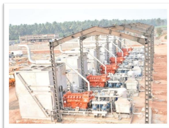
Gas Compression Station, GITL Tadepalligudem
