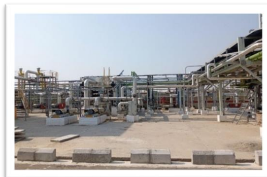
Compressed Bio Gas (CBG) Plant, HPCL – Badaun UP
